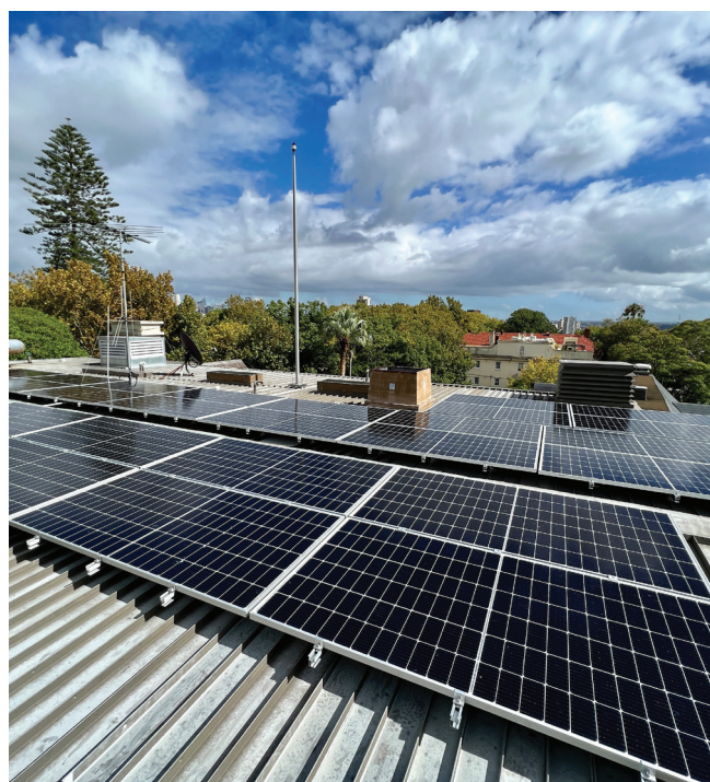
Solar panels on the Wolper's roof
