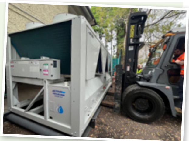
The temporary chiller being delivered
