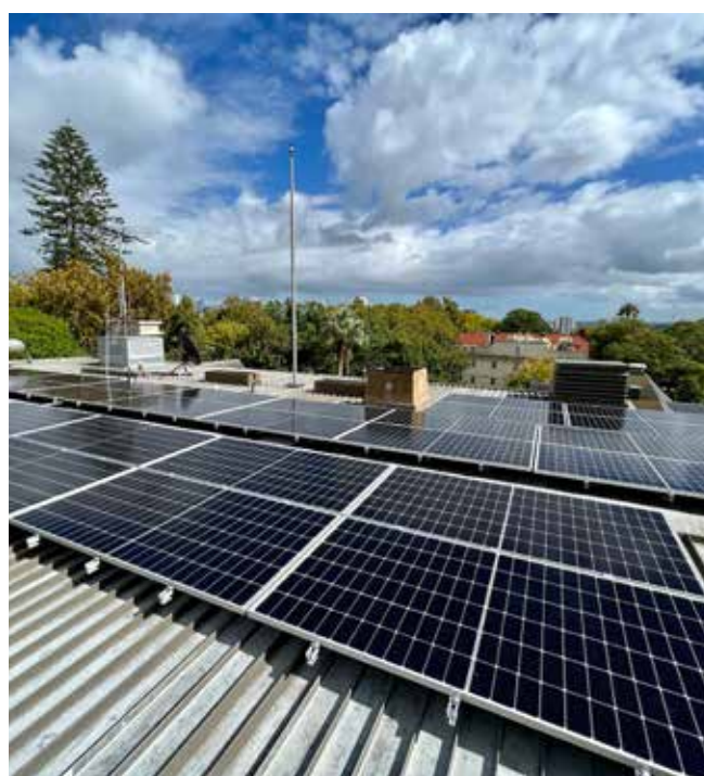
Solar panels on the Wolper's roof
